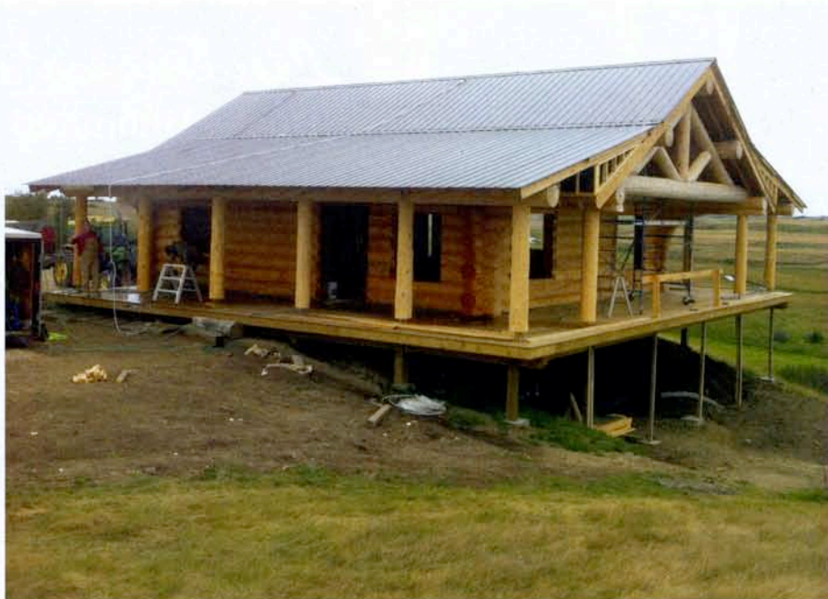
ABOVE SIP roofs are popular among log homebuilders. One reason is that in most cases, there is already a crane on site for lifting the logs. The roof panels on this log cabin were installed in three hours and then topped with metal roofing.
